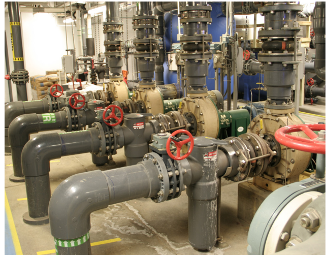
Four pump motors modulate flow control for NEWPORT AQUARIUM®'s 380,000 gallon shark tank.
