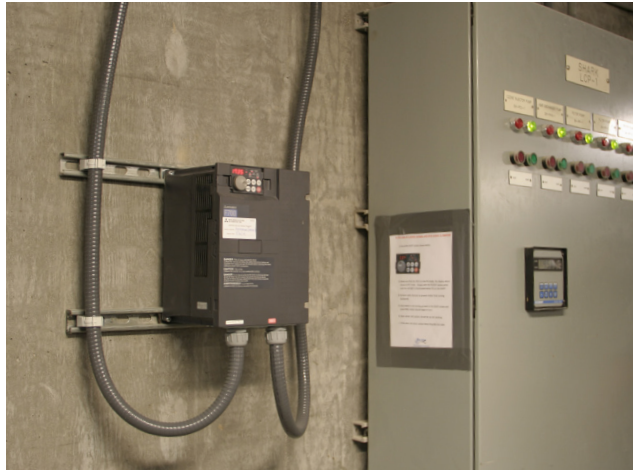
F700 Variable Frequency Drives control 25-horsepower pump motors for NEWPORT AQUARIUM®'s shark tank.
